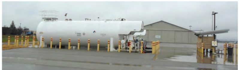
Fuel Storage Facilities
