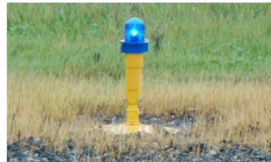
Medium Intensity Taxiway Light (MITL)
