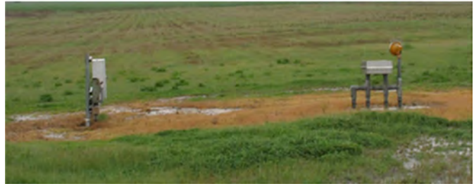
Runway End Identifier Light (REIL)
