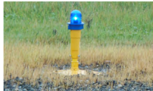
Medium Intensity Taxiway Light (MITL)
